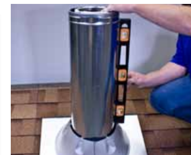
12. Add more chimney sections until chimney is at least 3 ft above roof, and at least 2 ft above any part of your house within 10 ft.
