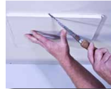
1. Drop a plumb line to center of stove flue collar. Mark center point on ceiling, and cut and frame a 14 1/2" square opening around this center point.
