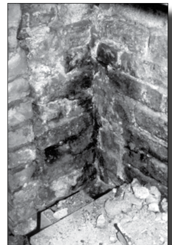
Debris at bottom of flue
