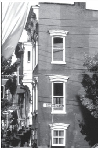
Wet exterior wall
