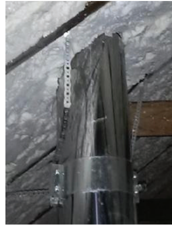
This example shows spray-foam insulation in direct contact with the chimney which is a serious potential fire hazard!
